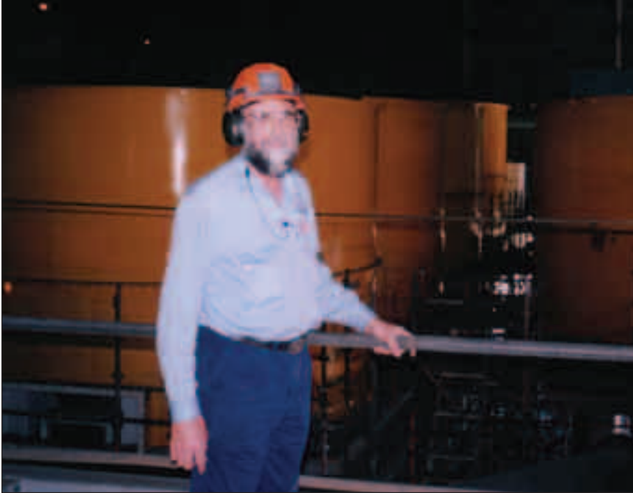
Impressive sight - Met Plants Construction Superintendent Fred Dunn inspects the installation of the Copper Concentrator's six new tank cells.
