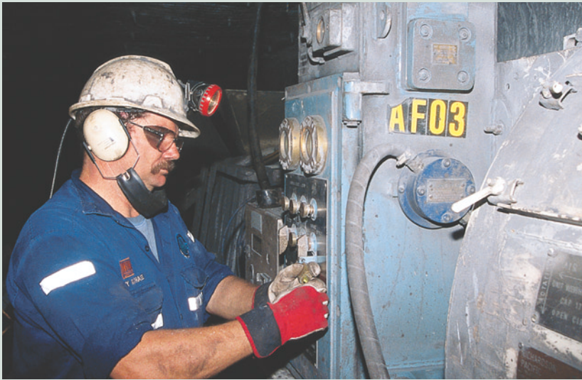
◀ Garry Kathage, Oaky Creek Development Crew Supervisor, inspects the auxiliary fan at the Oaky No 1 mine.
